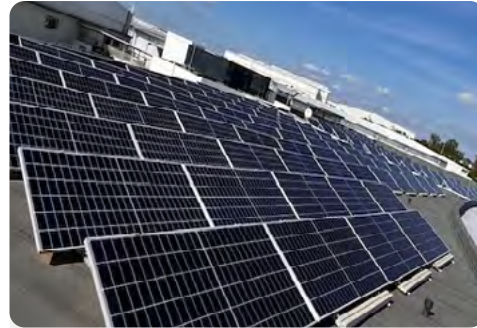
Photovoltaic system at VEGA South Africa
