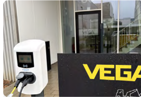
Electric vehicle charging station at VEGA Belgium
