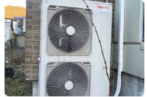
Heat pump at VEGA Norway
