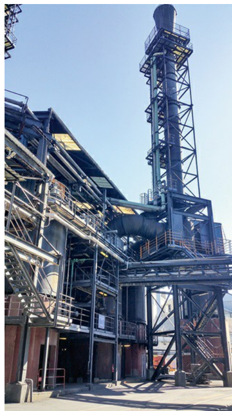
After the sulphating process, the first production phase of titanium dioxide creates highly challenging conditions for sensors.
