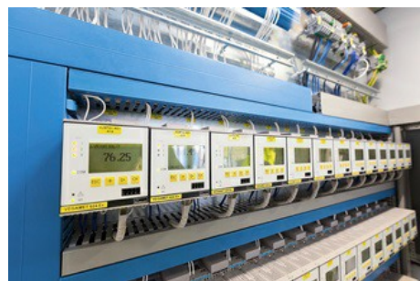
Control cabinet with VEGAMET 624 controllers for the underground solvent storage facility.
