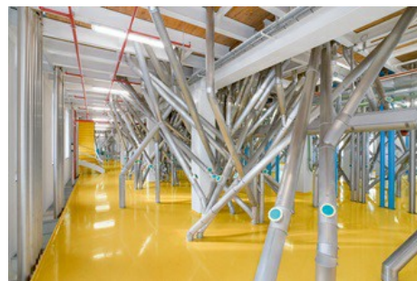
The piping network conveys the intermediate products to the roller mills. Every process step is comprehensively monitored during operation.
