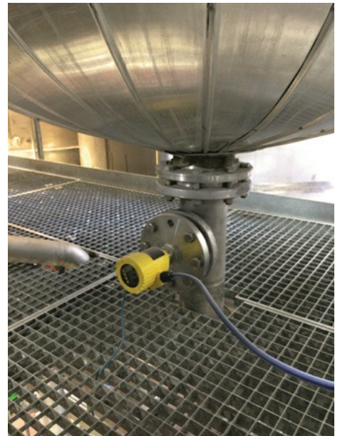
Electronic differential pressure measurement of a primary sensor in a distillation tank.
