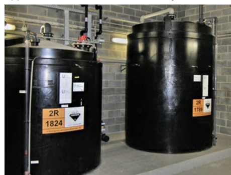
Chemical tanks for storing acids and alkalis.
