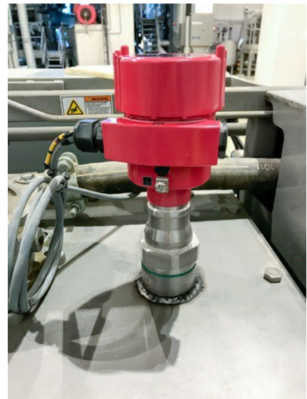
Notice that these VEGA sensors are not yellow, but the typical Progroup red.
