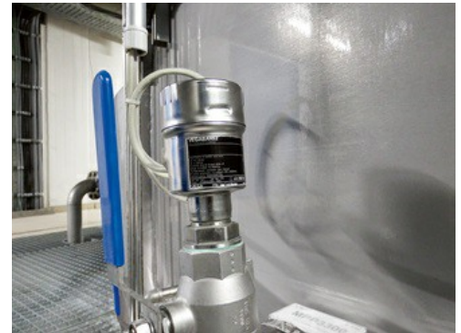
Measuring point with VEGABAR 82 and “Second Line of Defense”.
